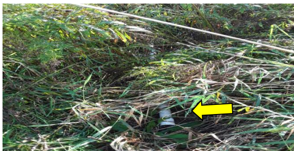
White PVC sewer line discharging waste to ground surface.
